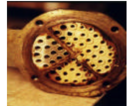
Heat Exchanger Before ED 2000
