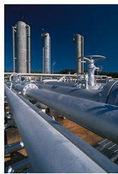
The ED 2000 was installed in a Gas Processing Facility in Texas
